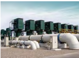
Fujairah Desalination / UAE
